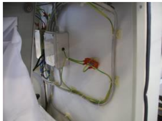
Earth connection during the maintenance operation
